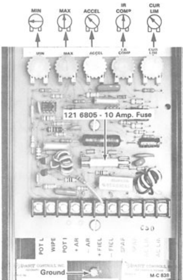
Figure 58 - SCR Drive Control Board Approximate Trim Pot Settings
